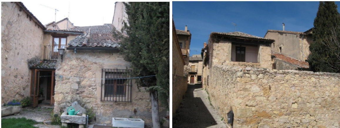
Fig. 4- Different views of the decks of the casona del siglo XVII used as an example in this paragraph. In the image of the left can be seen the solution of reddish segoviana mentioned
