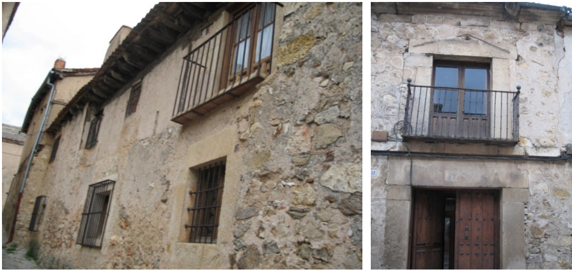
Fig. 2.- Aspect of the load-bearing walls of facade of the casona del siglo XVII that we are going to use as an example in this section.
